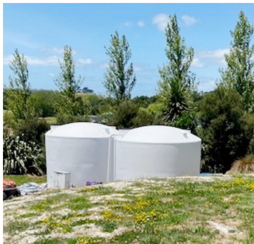
Water supply for the house
